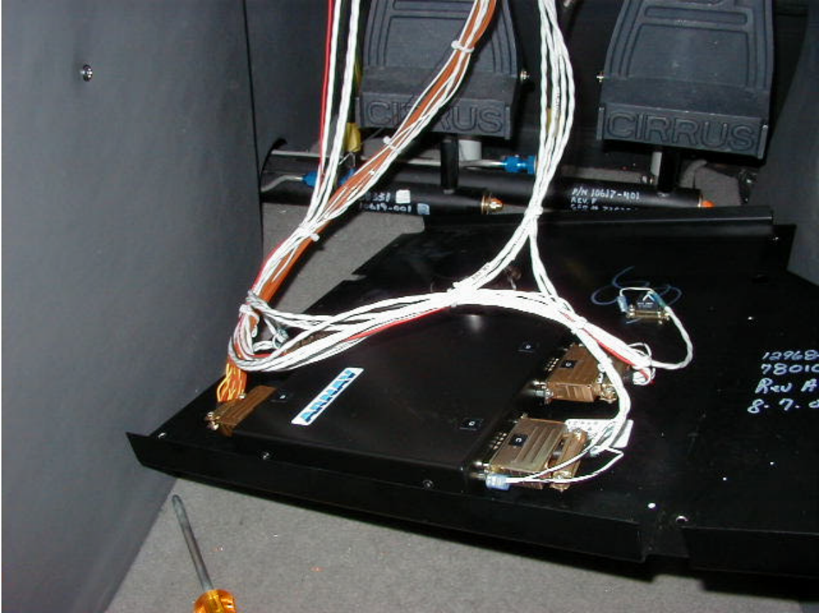
Kick Panel With EMM-35 and All Connections Final
